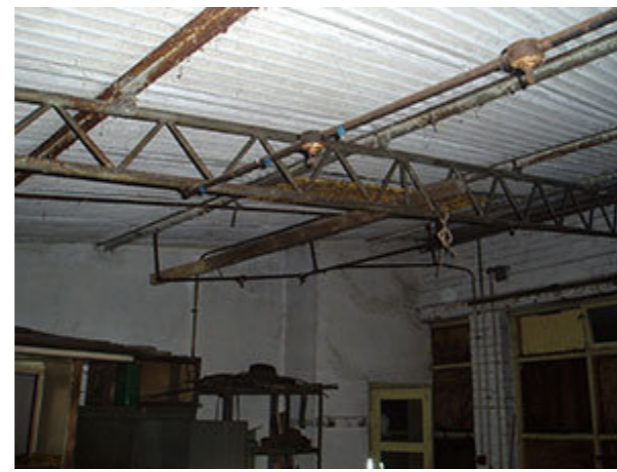
A closer look at the tubular steel roof trusses which are remarkably similar to the tubular chassis frames! Perhaps Charlie Toghill was involved in their manufacture. Maybe???
